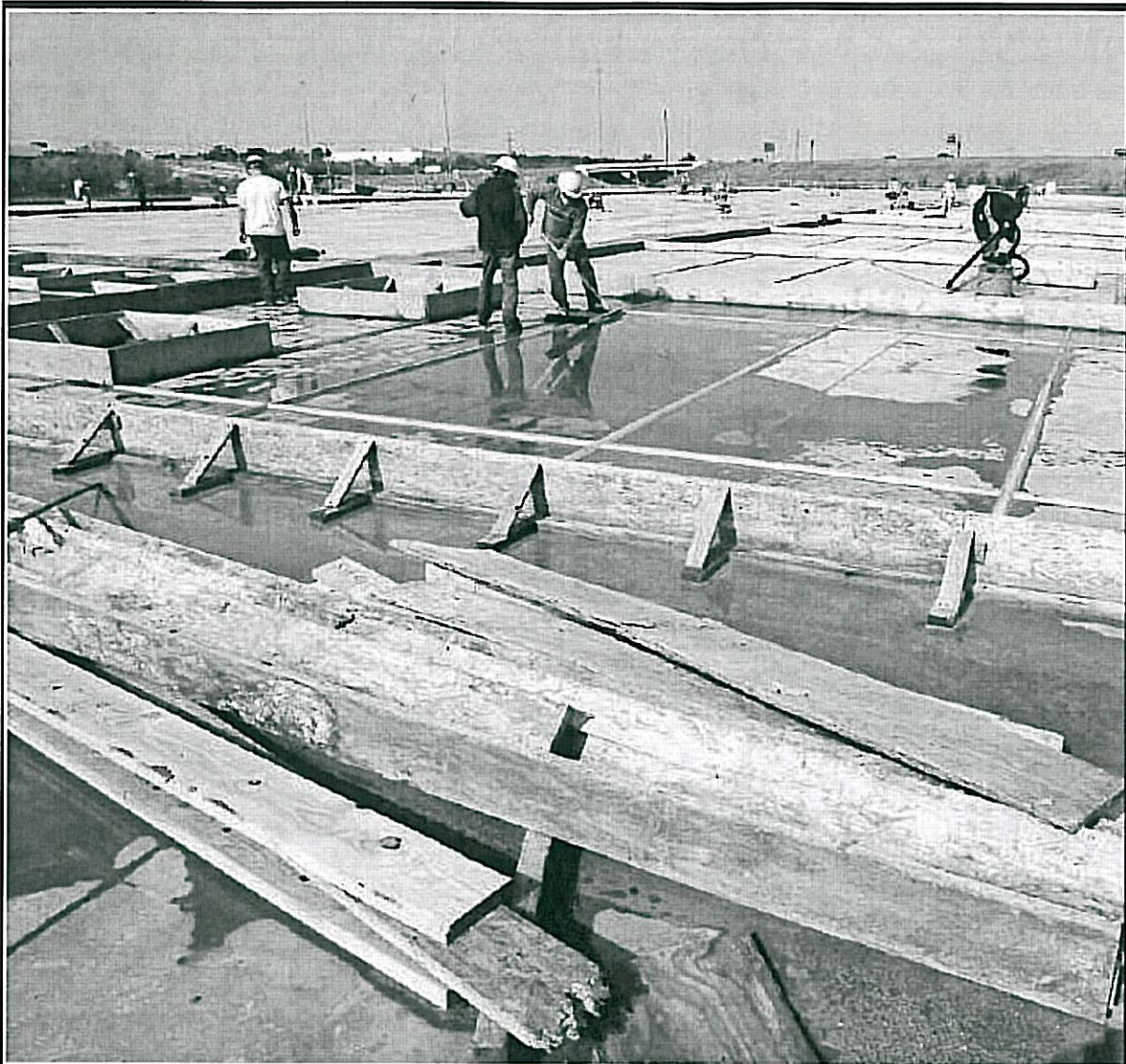
Gardner-Tanenbaum Group is developing Hefner Commerce Park on the north side of Hefner Road east of Interstate 35, where Capstone Construction Services is building a 100,000-square-foot warehouse-distribution center to be used partly by Kellogg Co. PHOTO BY PAUL B. SOUTHERLAND, THE OKLAHOMAN
